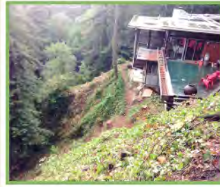
All trees cleared on this slope
